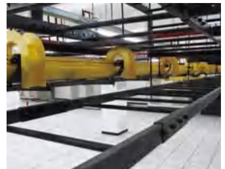
北京某机房施工实例 Construction practices in a machine room in Beijing
