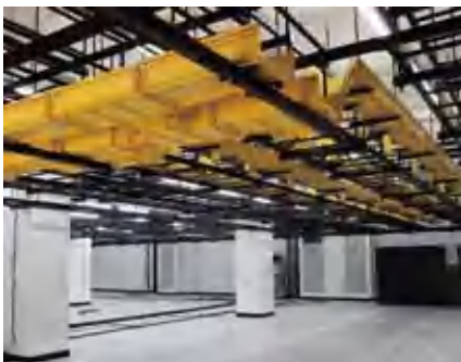
北京某机房施工实例 Construction practices in a machine room in Beijing
