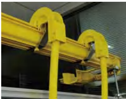
光纤槽道下引 Optical fiber channel downward
